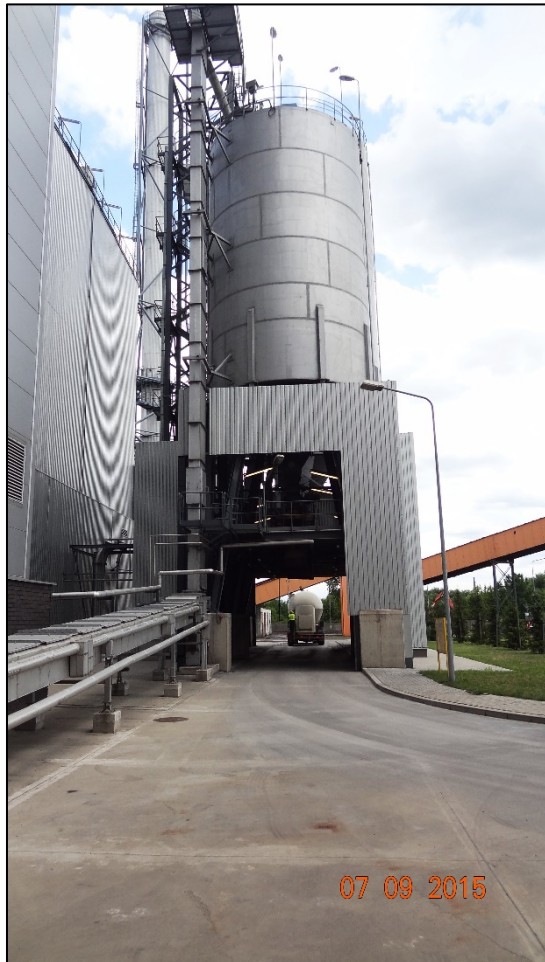
Figure 4-9: Bottom ash silo with truck loading facility
